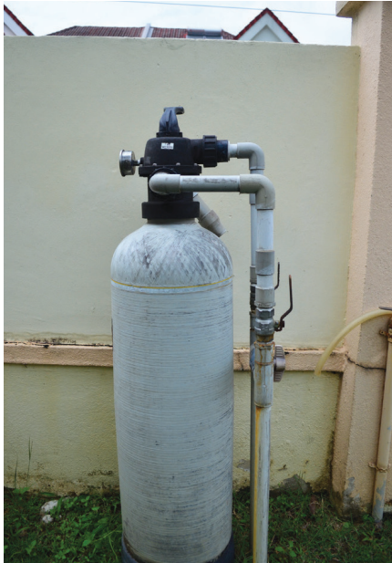
To ensure the health and wellbeing of the home's eight residents, and protect their water tank, the family installed Waterco's W300 high-strength water filter.
